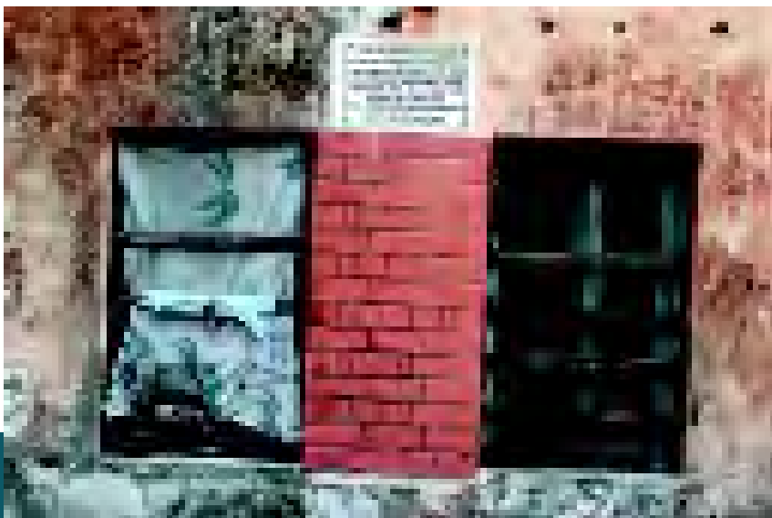
The irrigation inspection bungalow did not fulfill its intended function because the irrigation barrage (shown in facing page) became defunct one year after its completion as the Tinau River changed its course.
