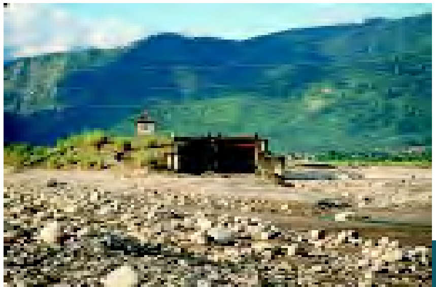
The defunct Tinau Barrage in Butwal. Shortly after construction the main channel on the Tinau River shifted, bypassing the barrage. As a result, the new irrigation system never functioned.
