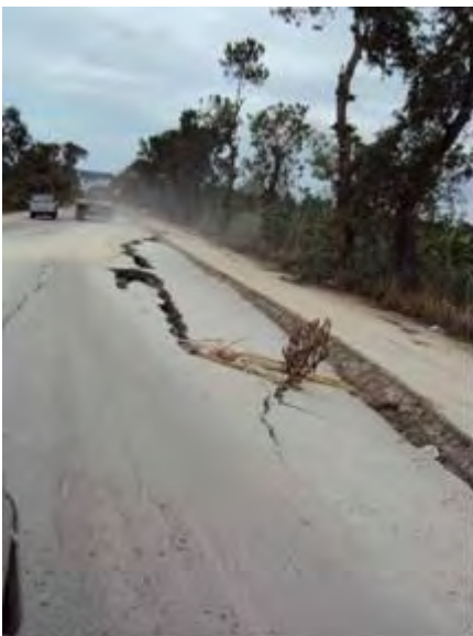
Transport infrastructure damage near Leogane.
