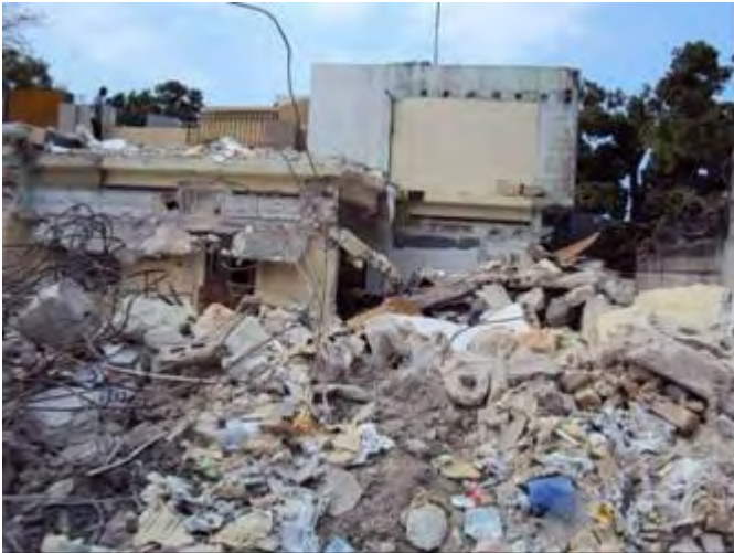
Rubble management challenges - mixed waste, debris and metal in PAP.
