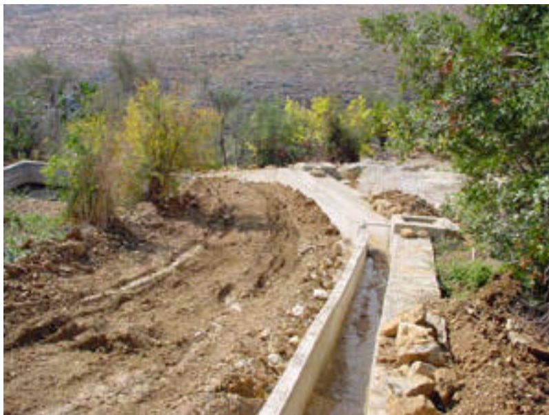
Photograph 5.2. Agricultural road on the Southern side of the parcel showing part of the waste water Network along with a storm water canal. This road ends at the Western edge of the land
