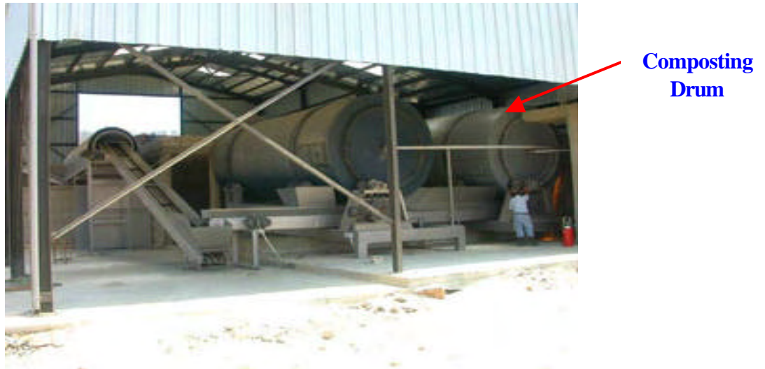
Photograph 3.1. Typical Composting Drums in Qleia.
