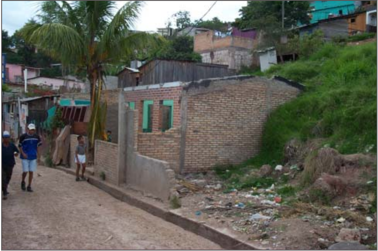
Figure 11. Toe of slump in neighborhood of Campo Cielo in Tegucigalpa. At the right of the photo, the toe of the slide mass is seen impinging against the row of houses.
