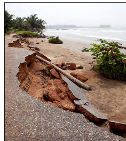
Figure 2: Washed feeder road along Ankobra beach
