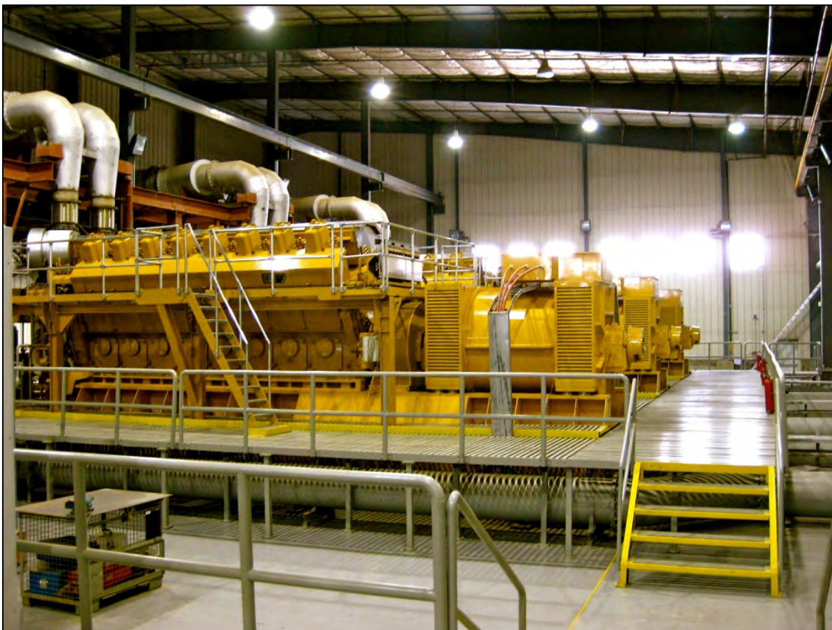
Generators in Tarakhil’s Block B remain idle because of a control system malfunction. (Photo by OIG, January 23, 2014)
