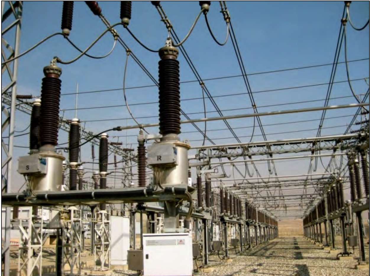
The substation at Tarakhil where circuit breakers and other equipment are used to connect the power generated at the plant to the grid. (Photo by OIG, January 23, 2014)
