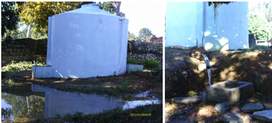
Figure 25: Leakage from Water Tank in Vondrozo
