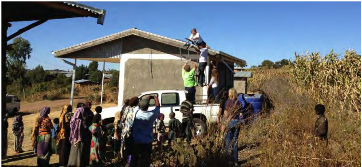
UC and HU students installing solar panels at the clinic while villagers watch.
