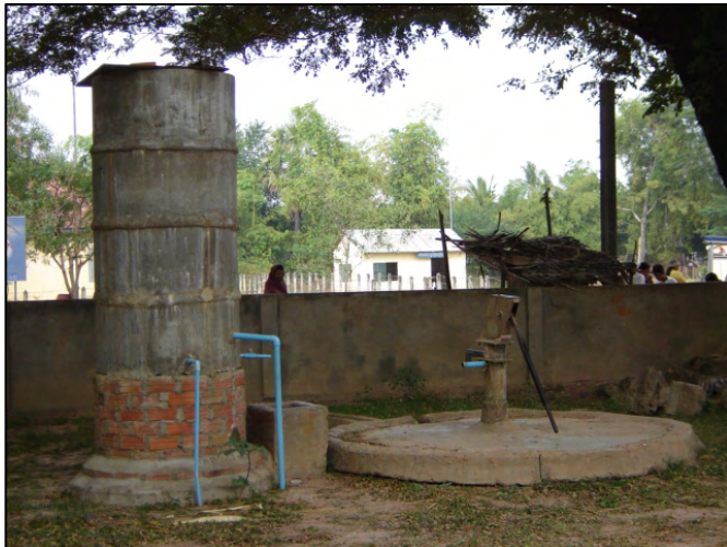
A locally constructed water system for providing clean water throughout the school
