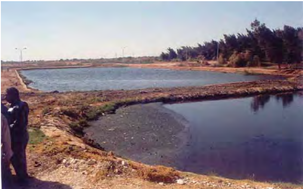
Figure 10. The existing Balat WWTP: An anaerobic pond, a larger facultative pond beyond it, and an irrigated grove of casuarina trees.
