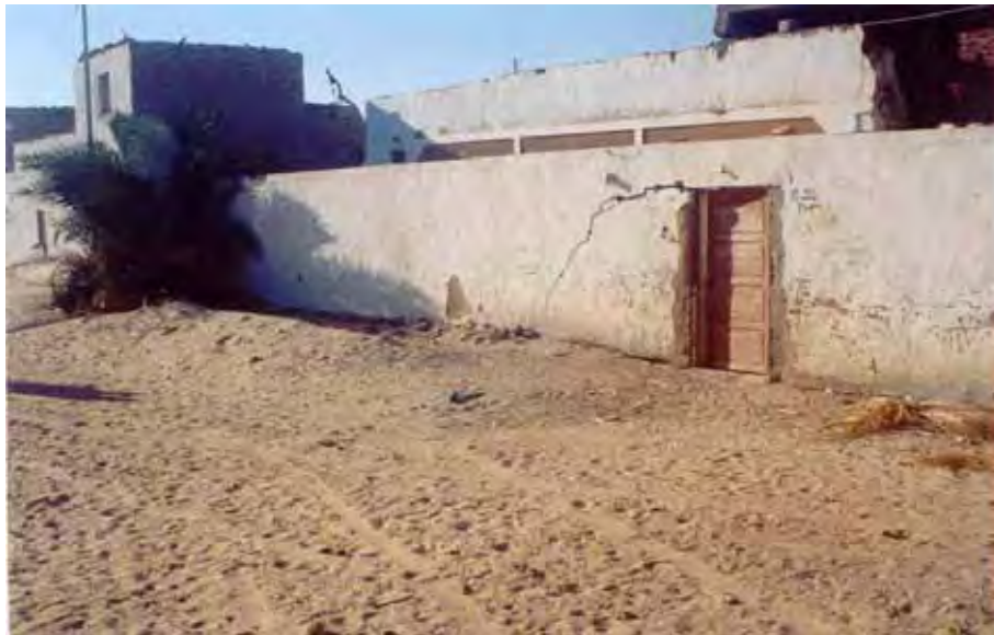
Figure 3. Structural damage to a wall from soil expansion due to a sewer leak.
