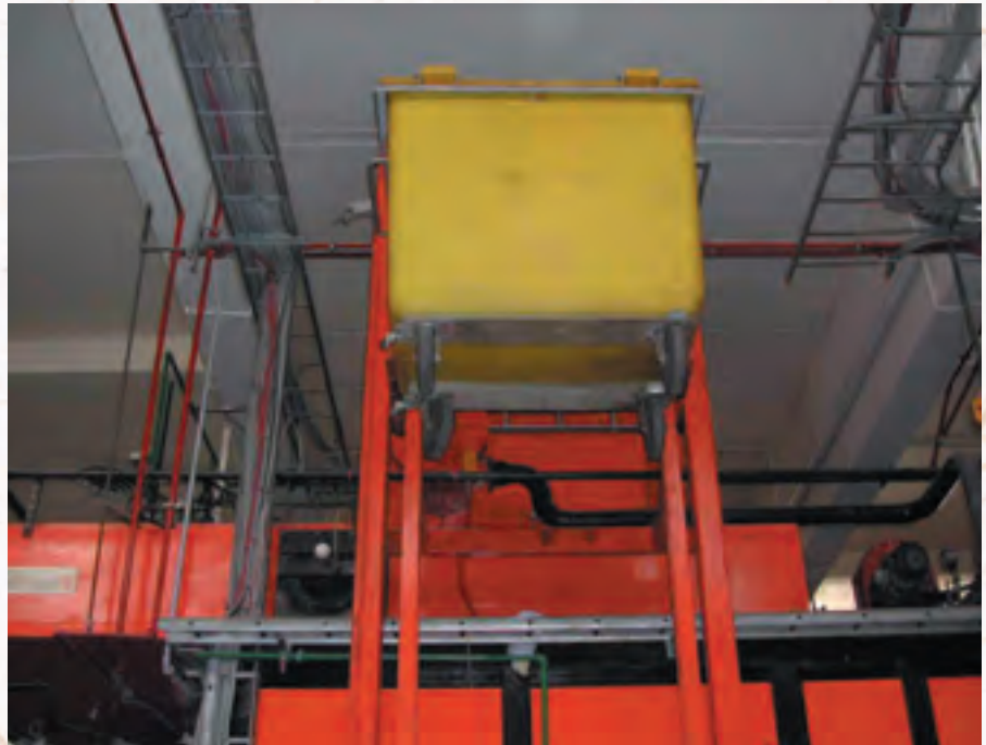
Lift for incinerator cart.
