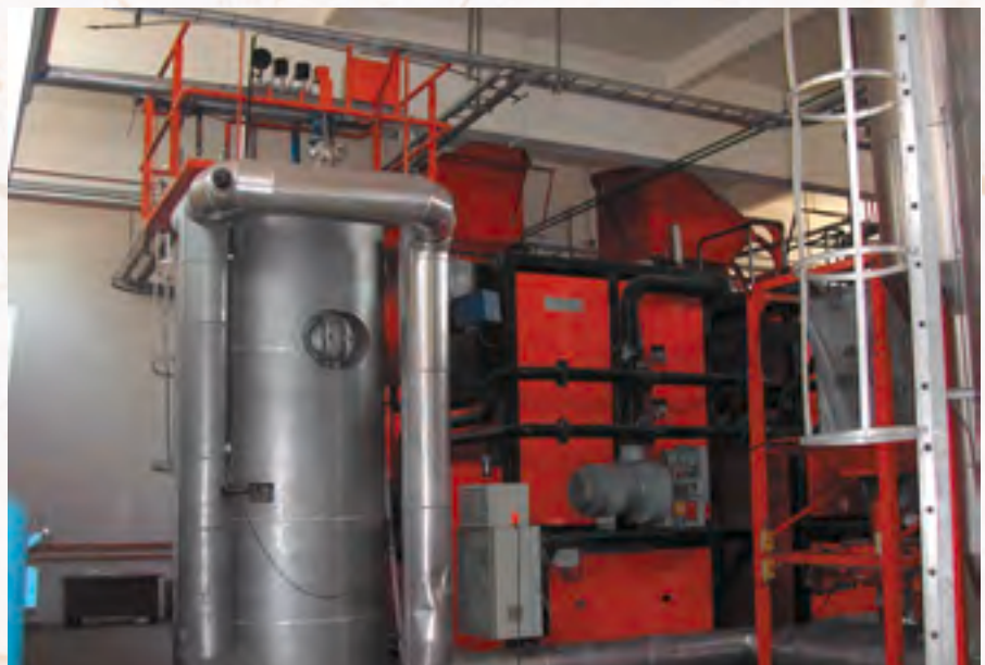
Medical waste incinerator, indoors.
