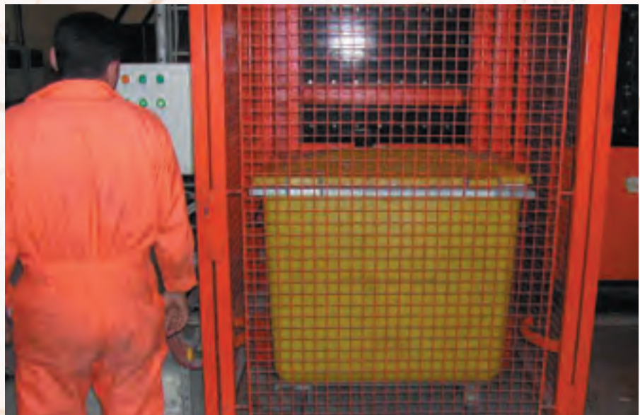
Incinerator cart handling system.
