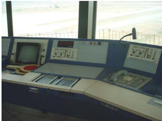
ATC Consoles – Phone System
