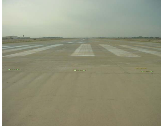
RWY 33R Threshold (lights)
