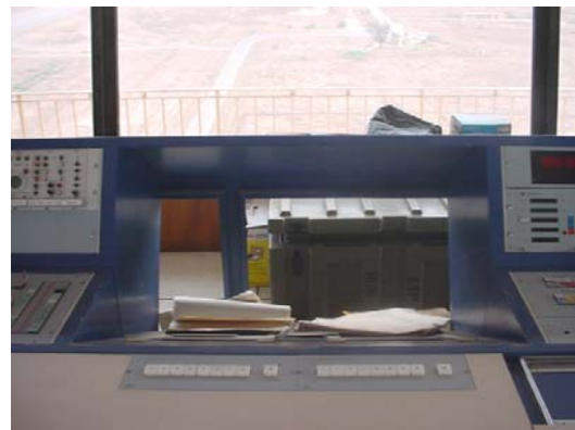
ATC Consoles – Missing Radar Display
