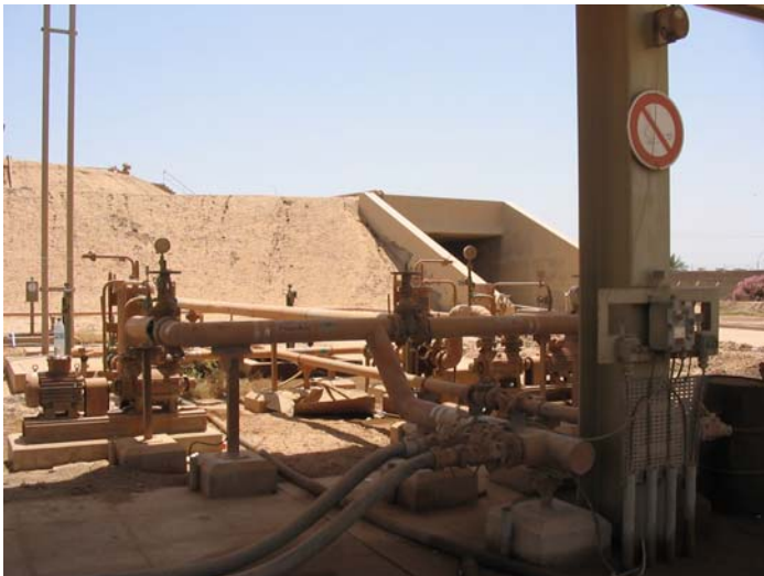
Fuel Farm – Tank Fill Pumps
