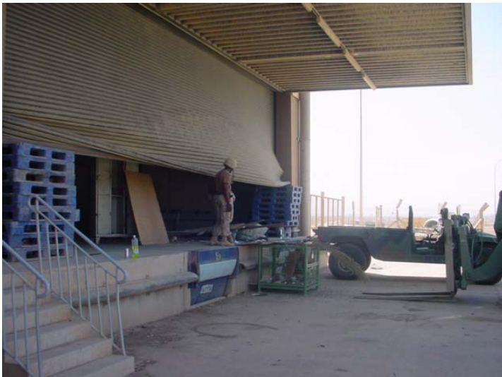
Damaged Roller Doors – Truck Docking Station
