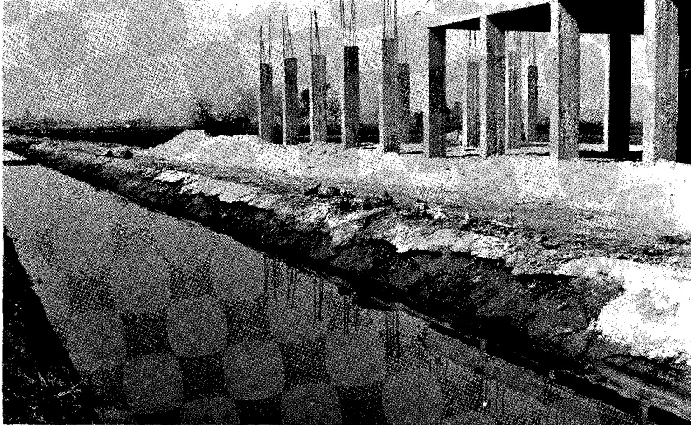
PHOTO 3 - BENI MAGDUL CANAL SHOWING BANK LINING FAILURE CAUSED BY EXTERNAL BANK LOADING.
