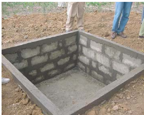
Curing chamber or pit
