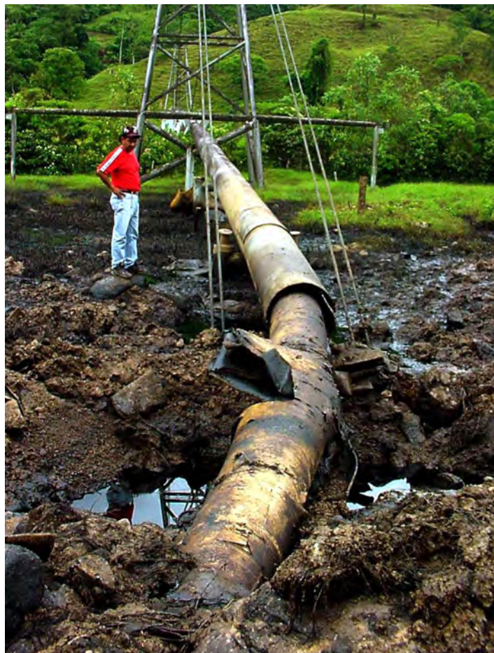
A man surveys the damage done to the Cano Limon-Covenas oil pipeline after it was bombed by FARC guerillas in August 2001. (Efrain Patino,AFP)
