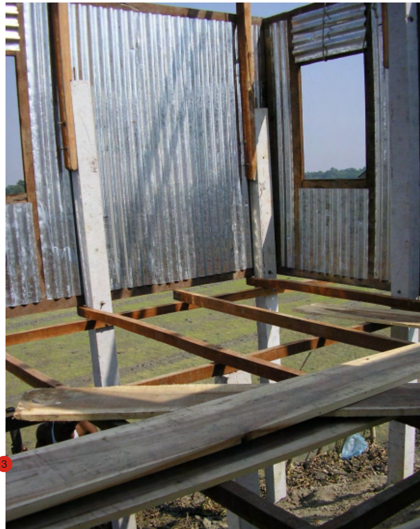
Fig. 5.11 Stilted houses near Mawa 1. Example of a stilted house 2. Stilted house being built 3. Stilt construction detail showing connection between RC Post and timber members
