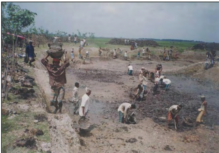
About 1.8 million person days of work was created through manual excavation of silted up wetlands
