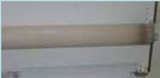
Bulbs and ballast burn out
