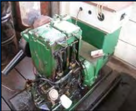
On site generator: 10 am – 2 pm
