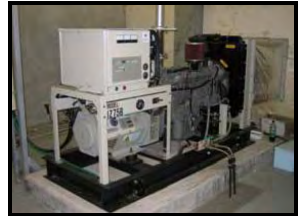
75 kVA backup generator
