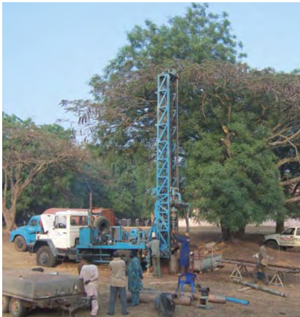
Workers build a water system for a Nigerian hospital with the help of a VfP volunteer.
