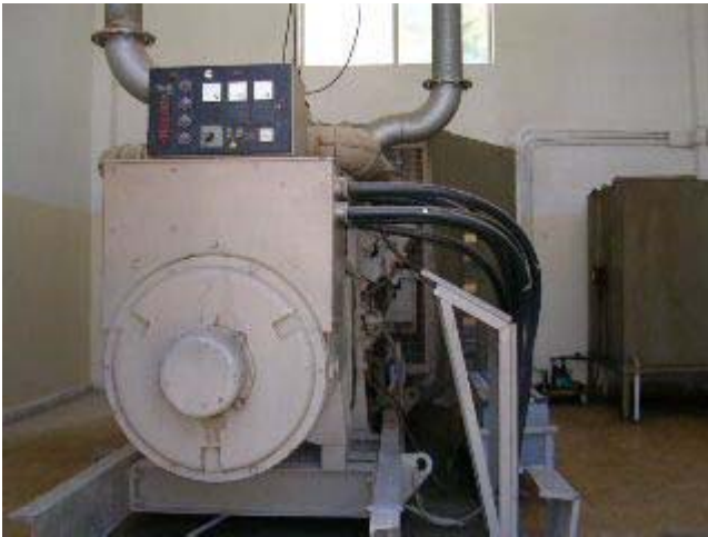
Figure 6: Main Pumping Station Engine-Generator Set
