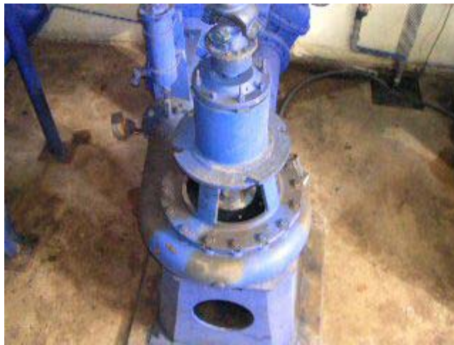
Figure 5: Existing Pumps in the main pumping station
