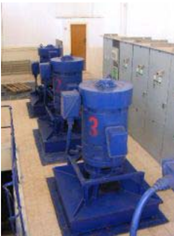
Figure 4: Existing Motors in the main pumping station
