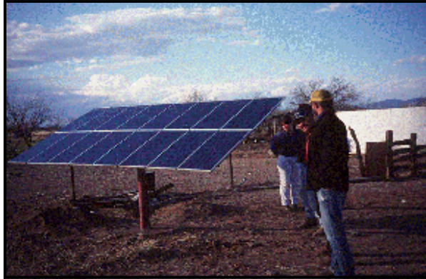
Figure 3. PV pump at Rancho Jeromin in Chihuahua.
