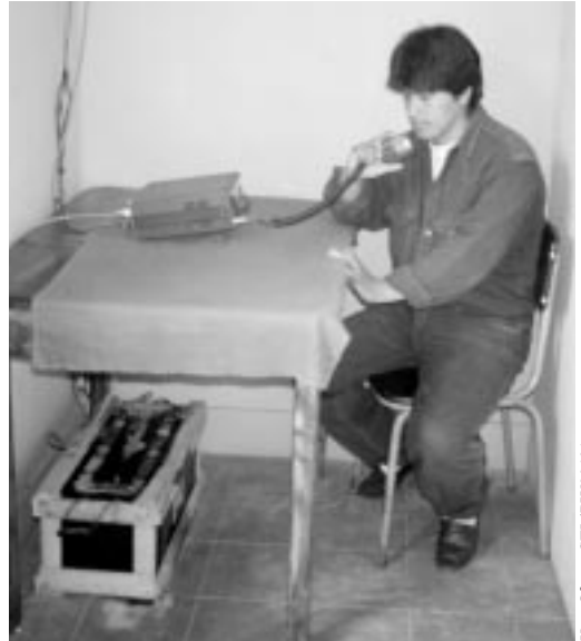
Figure 1.3. A PV powered radio is used by health staff at Clinica El Pallar to request technical or logistical assistance and to report on significant health risks in the region.
