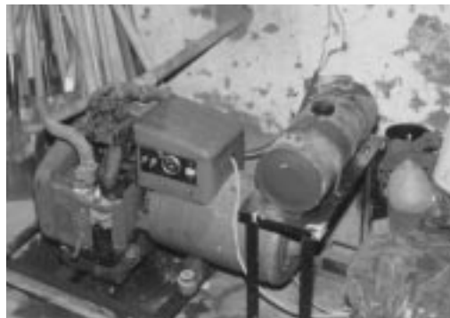
Figure 3.8. Typical generator at an isolated mountain school. Teachers and custodians generally have no training in the maintenance and operation of these units.
