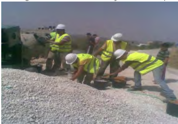
Workers hand-mixing concrete as part of the labor-intensive approach on EJP. If a machine were used, only one person would have employment as the machine operator.
