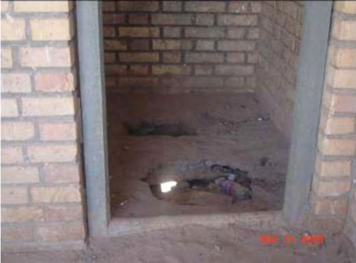
Broken toilets in the Laisa Islam Qila school in Herat province. (Photo by KPMG Afghanistan.)
