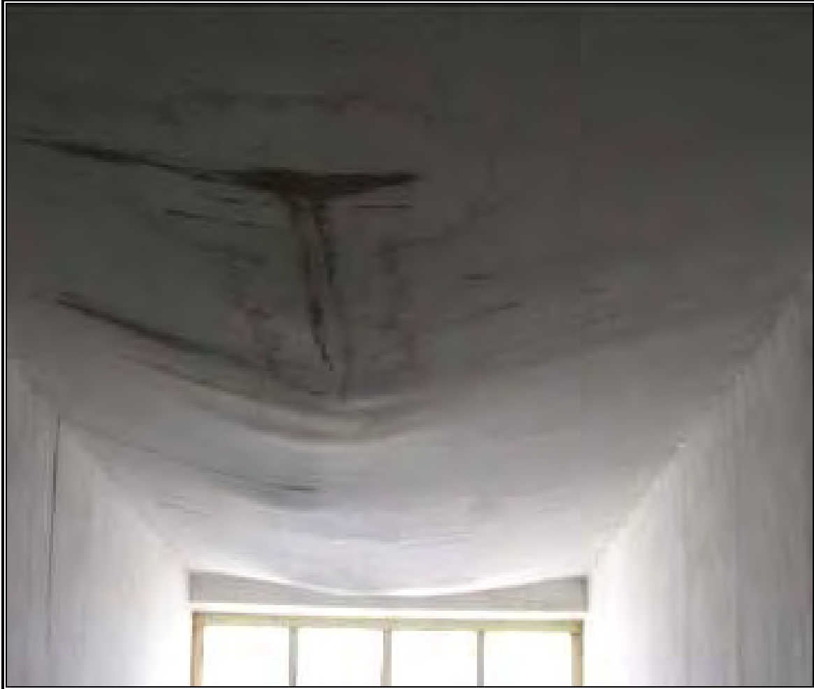
Ceiling at Del Hassain Primary School in Balkh province, which shows evidence of water damage and a defect in the roof. (Photo by KPMG Afghanistan.)
