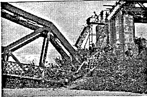
June 1994: Pedestrians climb up and down ladders at fallen span; others wait their turn. [Photo: L.Toth]
