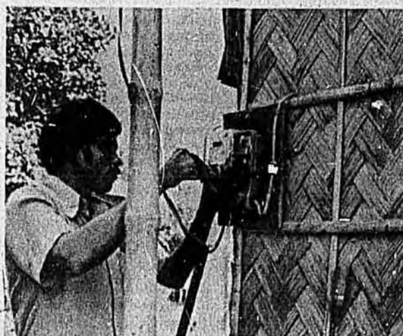
A village electrician on the job. Some 4000 rural youths are working in the PBSs as free lance village electrician.
