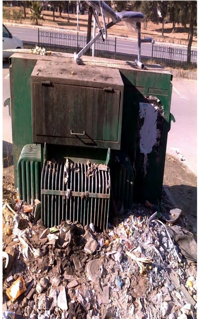
Figure 2.3.b. Pad mounted transformer.
