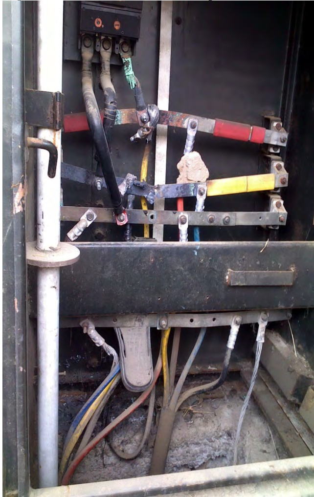
Figures 2.3 a. LT transformer compartment
