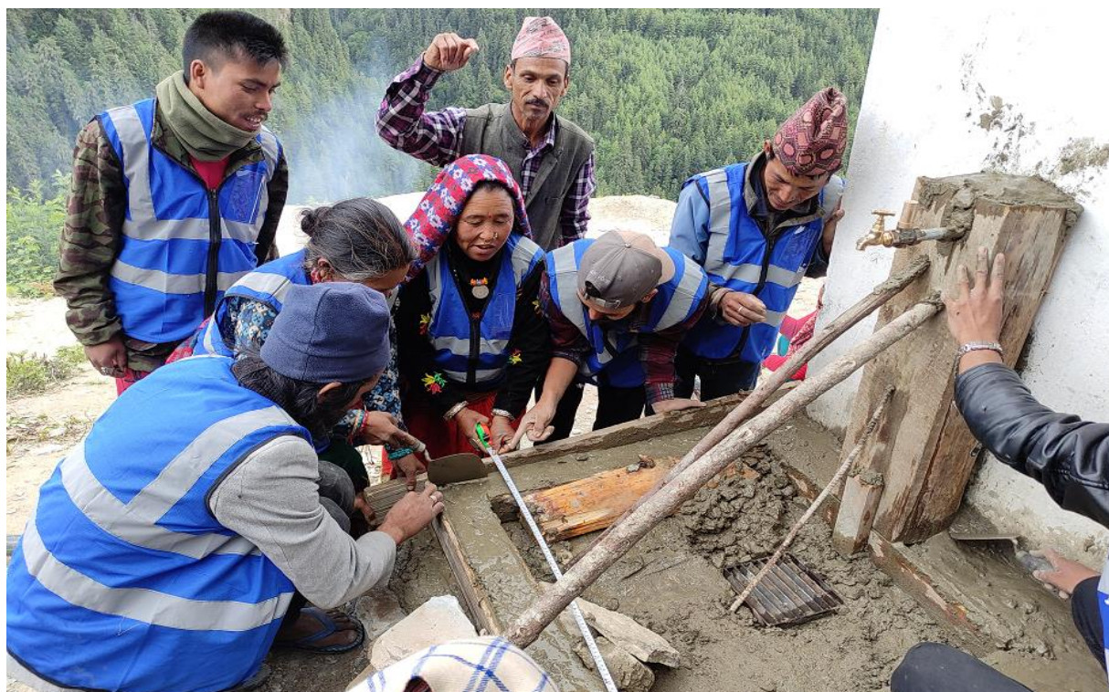
Photo: In the center of the image, [REDACTED] measures the slab using a tape measure during a practical session of village maintenance workers' training in Mugu
