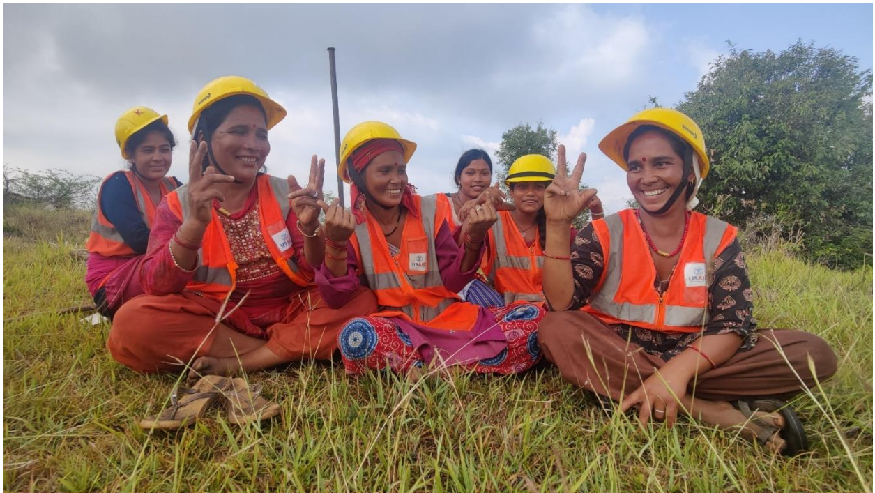
A group of women community members taking a photo-break after digging trench for pipeline in Pokharikanda Water Supply Scheme, Barahatal Photo Courtesy: ©Ramesh Dhakal
