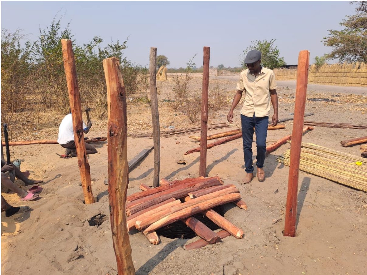
PHOTO CREDIT: [REDACTED], USAID EXPANDING WASH: USAID EXPANDING WASH PROJECT STAFF ENG. [REDACTED] WORKING COMMUNITY MEMBER TO CONSTRUCT A MODEL TOILET IN NALOLO DISTRICT
