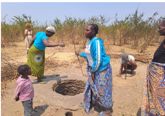
Photo Credit: Mutinta Nhandu. Pictured: Residents of Kaunga Luweti constructing model Baruto toilet.
