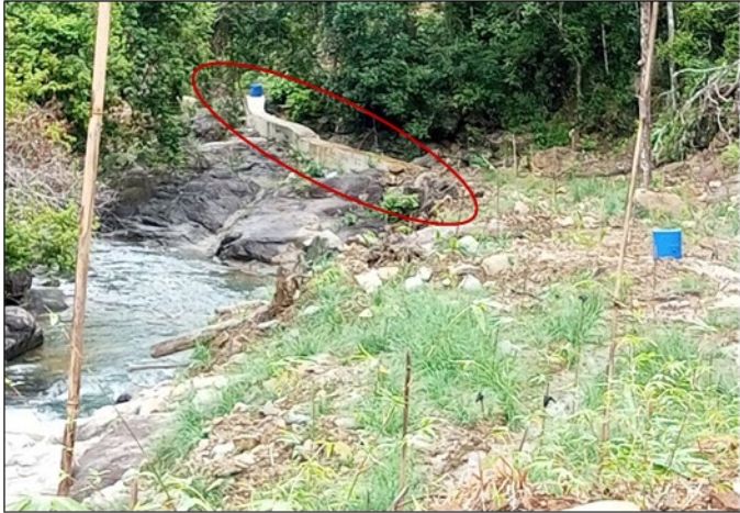
PPCWD- Lapu lapu Transmission Pipeline restored with concrete pipe encasement after typhoon Odette, SW TA climate resilient structure.
