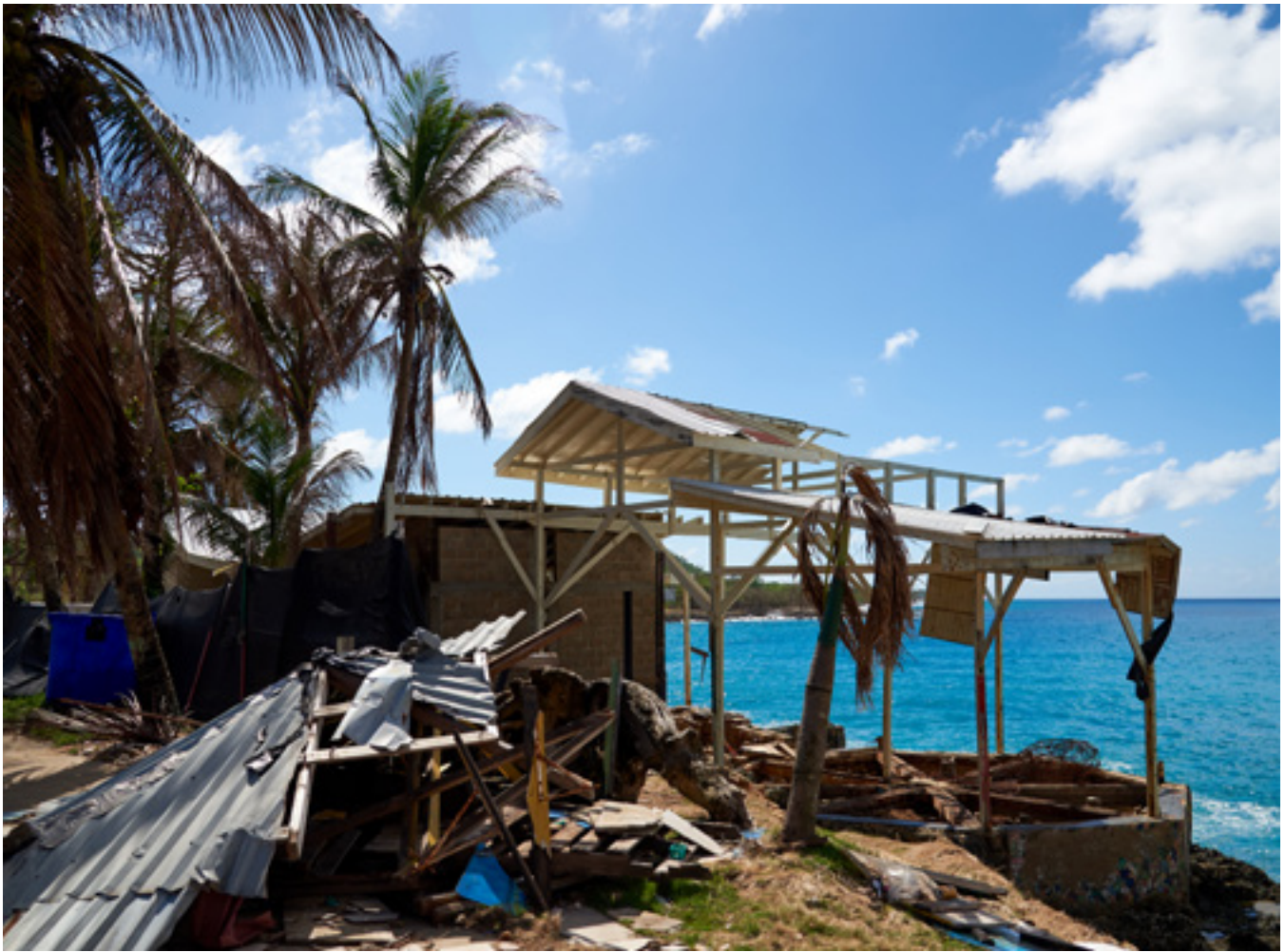
Providencia Island rebuilt its infrastructure damaged by Hurricane Iota using the Energy Master Plan. © EGT, Adobe Stock.
