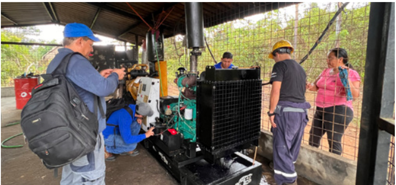
Regional operator and SURE diagnose non-operational diesel generators installed by the municipality in Zancudococha community. © Tetra Tech for USAID.
