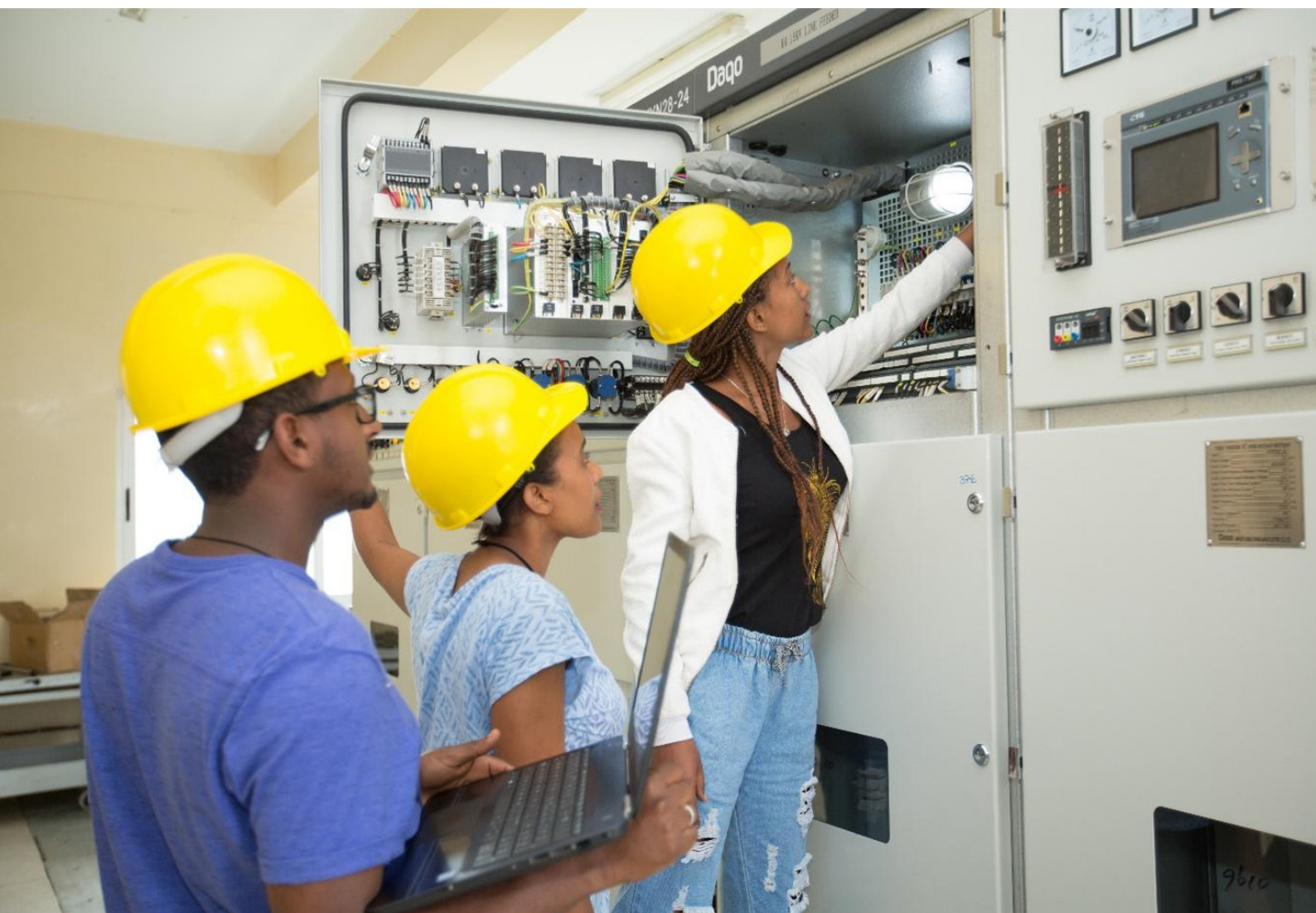
Staff at EEU performing equipment inspections with EAEP's utility-turnaround team. Photo credit: EAEP
