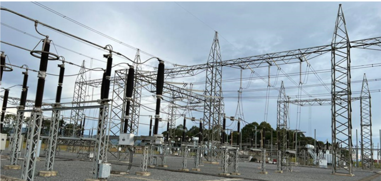
The 200 kV high-voltage alternating current Mawakibeta substation is critical for connecting Mbeya in southwestern Tanzania to its neighbors—Zambia, Malawi, and DRC—through a cable passing under Lake Tanganyika. Photo credit: EAEP
