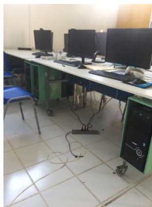
Curimana. Loose electrical connections
