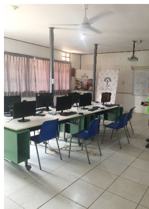
Campo Verde. Loose electrical connections. High presence of children.
