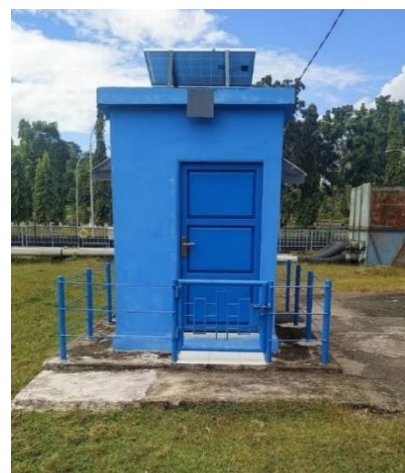
A typical water quality monitoring Onlimo system installed in Mamminasata's intake facility area in South Sulawesi.
