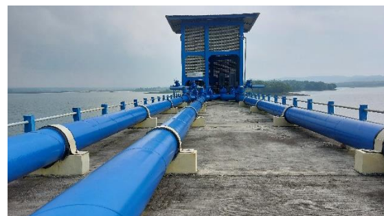
The Intake of SPAM Regional Wosusokas is located in Wonogiri Multipurpose Reservoir. The intake has been constructed in year 2019 and has capacity of 1.450 lps.
