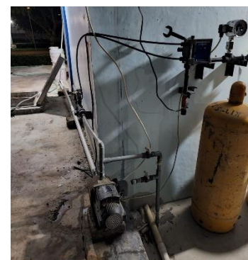
Chlorination system with pump dosing at PDAM Tangerang District, poorly maintained installation
