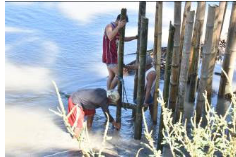
Stabilizing riverbanks for resilient coastal communities. Community members install bamboo dikes for riverbank stabilization.
