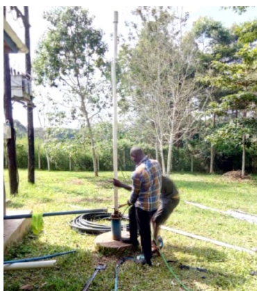
Figure 1. Retrieving the uPVC OD63mm riser pipes prior to test pumping (field photo from Nkoni WSS)
