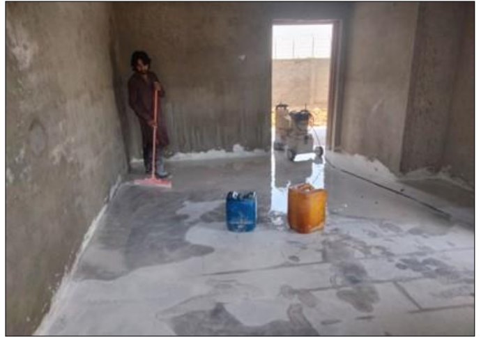
Photo 04: Construction work in progress at residential quarters – 132kV Grid Station Jandola, FR Tank
