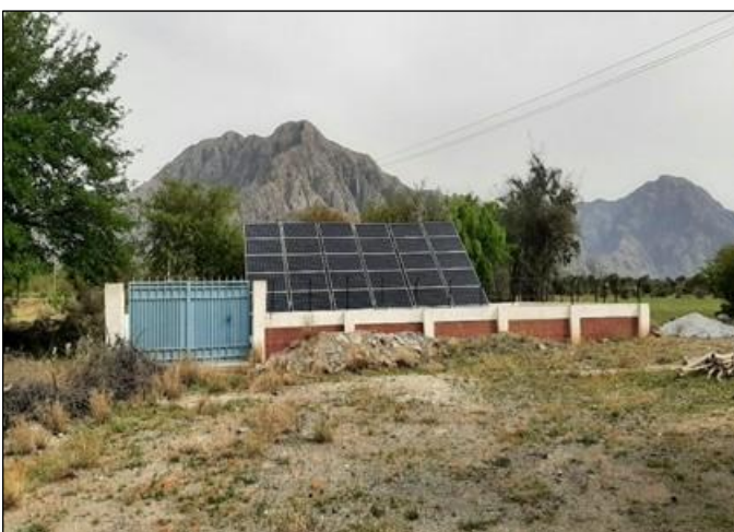
Photo 05: External view of solar panel compound – DWSS Mohra Mettai Baizai, Mohmand
