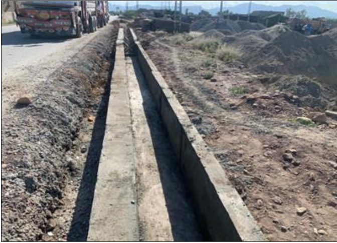
Photo 01: PCC side drain is in progress at RD 1+200 – Bara to Mastak Road, Khyber
