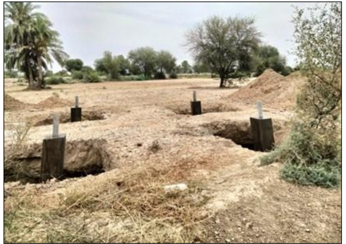
Photo 02 Stub foundation of T # 164 E in Re-routing completed. (Pkg # 04) – 132kV Transmission Line Pezu-Tank-Jandola, FR Tank
