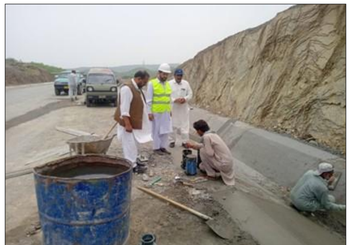
Photo 06 Casting of concrete cylinders for PCC side drain at RD 7+462 – Jamrud Bypass Road, Khyber
