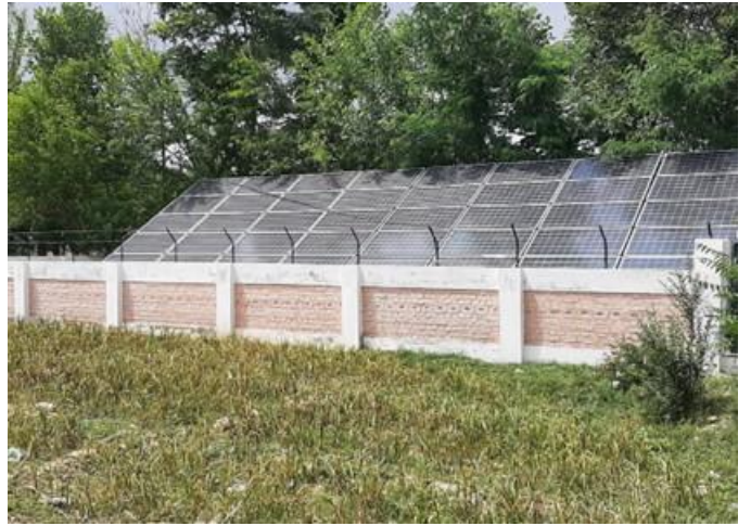
Photo 10: Solar panel compound completed – IWSS Khair Abad, Bajaur
