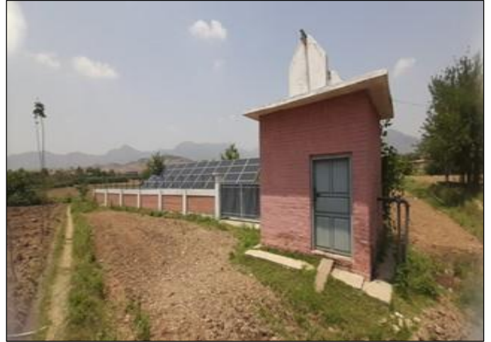
Photo 02: External view of pump house and solar panel compound – IWSS M. Zahoor, Mohmand
