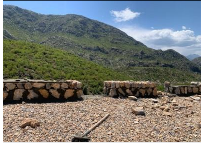
Photo 02: Parapet walls is in progress from RD 27+115 to RD 27+130 – Bara to Mastak Road, Khyber
