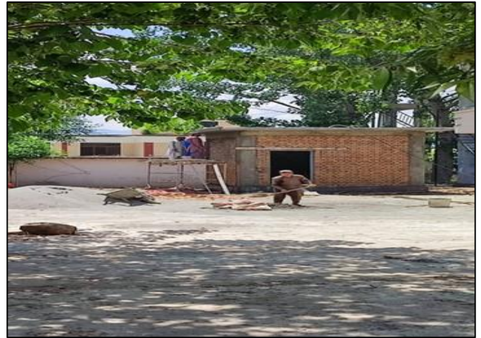
Photo 08: Construction works in progress without PPEs – Tehsil-Level Government Complex, Swat
