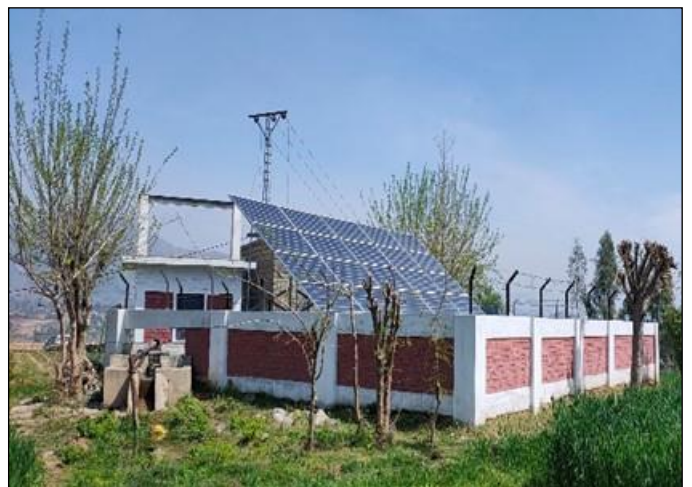
Photo 12: Solar panel compound completed – IWSS Umaria 2, Bajaur
