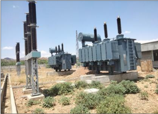
Photo 03 Placement of 02 Nos. 20/26 MVA Power Transformer completed – 132kV Grid Station Jandola, FR Tank
