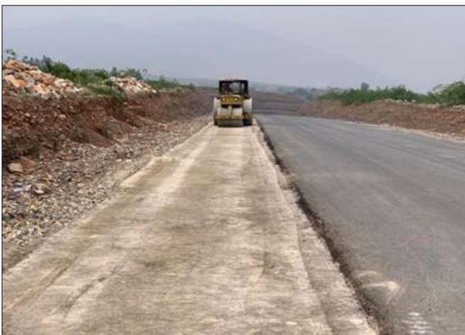
Photo 05: Compaction of water bound macadam on shoulders is in progress from RD 4+500 to RD 4+550 – Jamrud Bypass Road, Khyber
