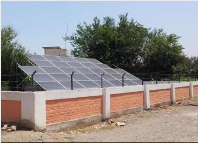
Photo 01: Solar panel compound – DWSS Ghariza I Jamrud, Khyber
