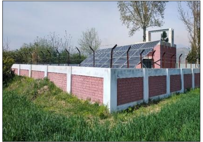
Photo 08 External view of solar panel compound – IWSS Dabdaboo, Bajaur
