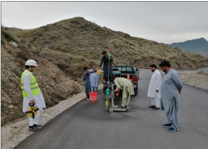
Photo 03: Coring of asphalt wearing course at RD 8+250 – Ghiljo to Dabori Road, Orakzai
