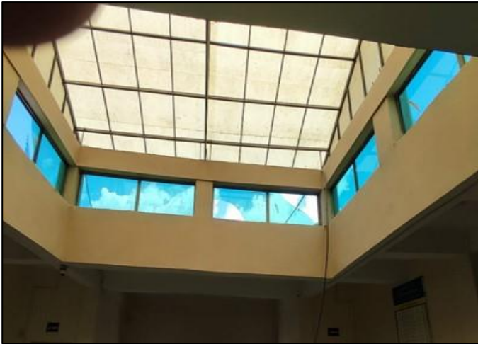
Photo 07: Shatter glass with damaged windowpanes at the District Government Building – Tehsil-Level Government Complex, Swat
