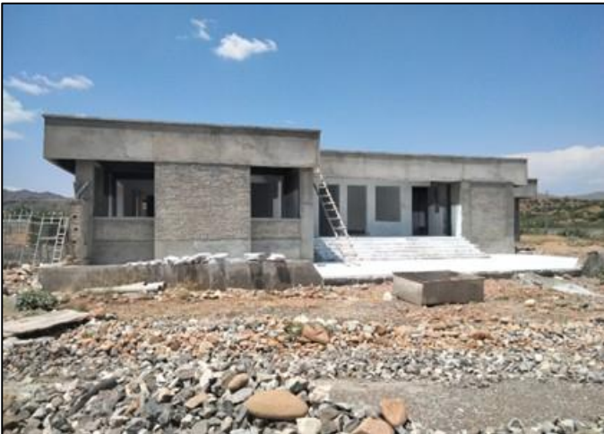
Photo 05: External view of control house building – 132kV Grid Station Jandola, FR Tank
