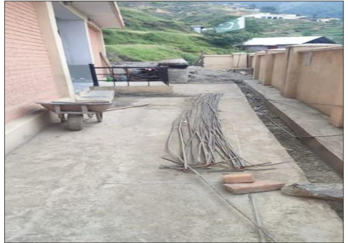
Photo 04: Steels bars are staked improperly in courtyard of the school – GPS Shandal, Swat
