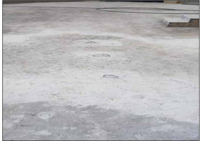
Photo 02: Manhole steel hooks to be bent to prevent tripping hazards – GPS Pansat, Swat
