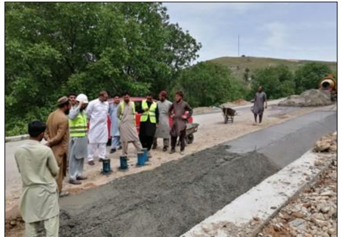
Photo 04: PCC for side drain and shoulder from RD 14+225 to RD 14+265 is in progress – Ghiljo to Dabori Road, Orakzai
