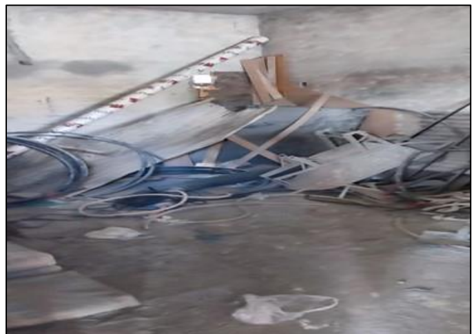
Photo 06: Improper stacking of material – Tehsil-Level Government Complex, Swat
