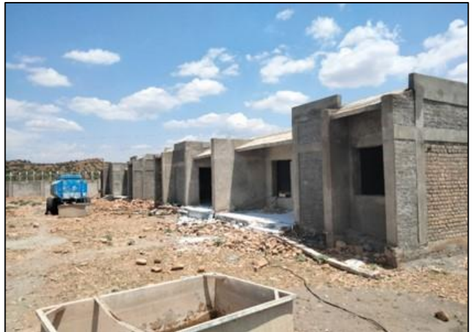
Photo 06: External view of Type IV Quarters – 132kV Grid Station Jandola, FR Tank
