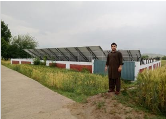
Photo 03: Solar panels compound completed – DWSS Bai China Khar, Bajaur
