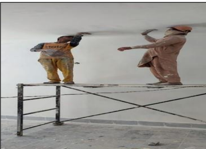
Photo 05: Paint works in progress without PPEs at Category B Residences – Tehsil-Level Government Complex, Swat
