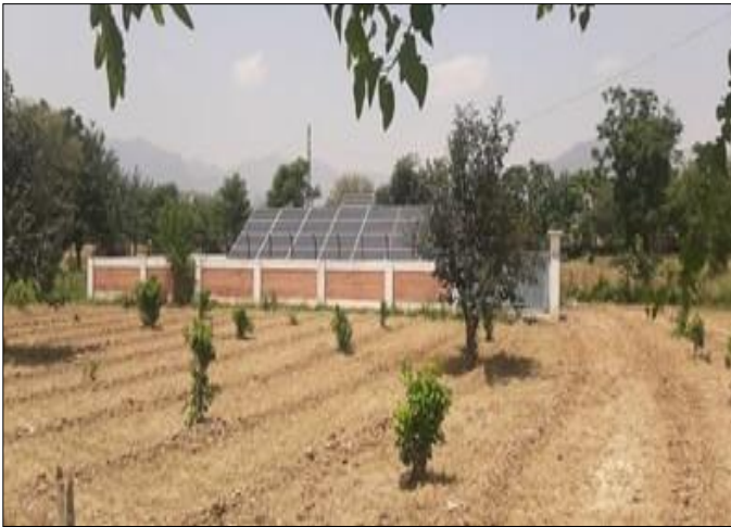
Photo 03 External view of solar panel compound – IWSS M. Hayat, Mohmand
