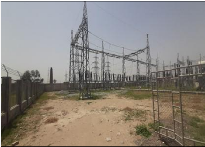
Photo 01: Switchyard electrical equipment installed at 2 x Line bays at Tank Grid Station – 132kV Transmission Line Pezu-Tank-Jandola, FR Tank
