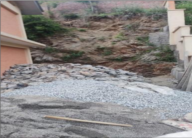
Photo 03: Construction material and debris are staked improperly – GPS Shandal, Swat
