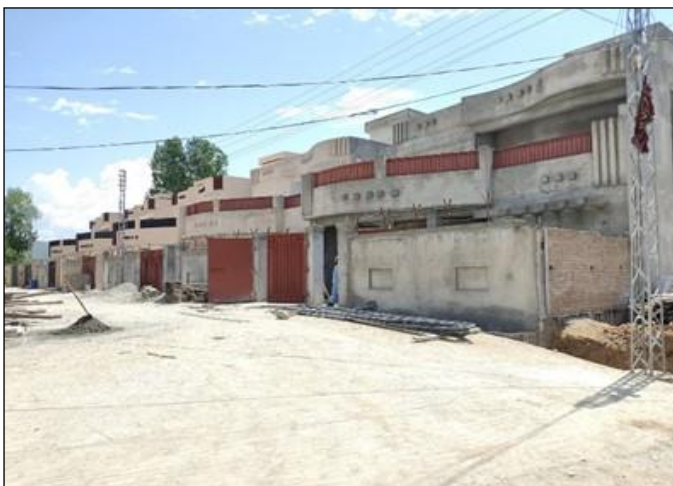
Photo 16. Construction view of category B residences No 6 to 10 – Tehsil-Level Government Complex, Swat
