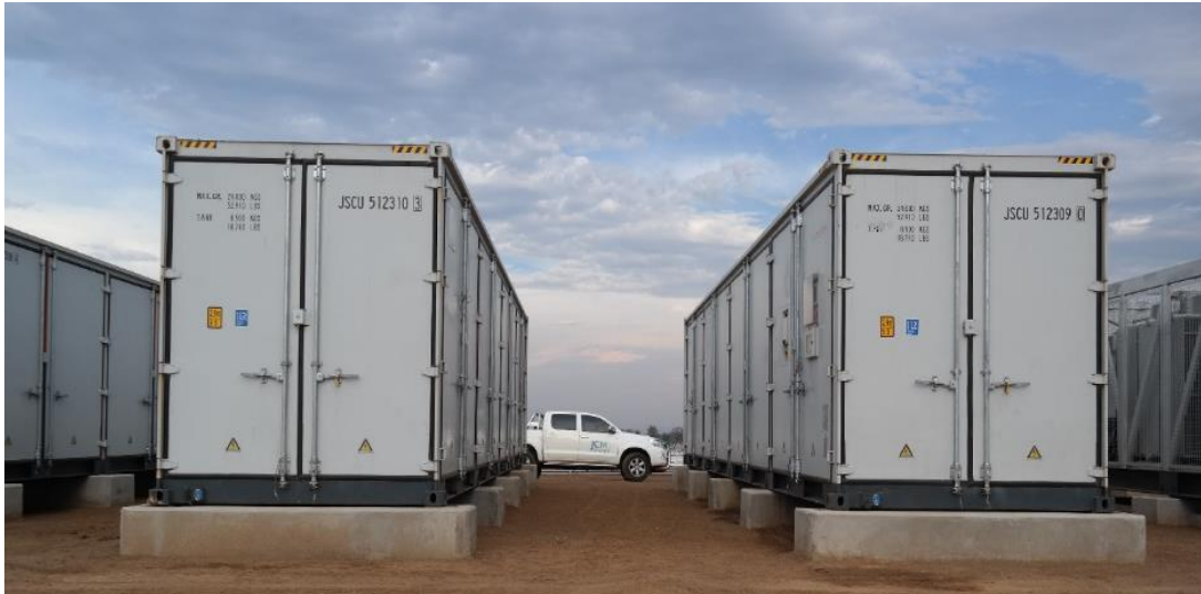
The 20 MW Golomoti Solar PV and Battery Energy Storage Project battery containers. Photo: JCM Power
