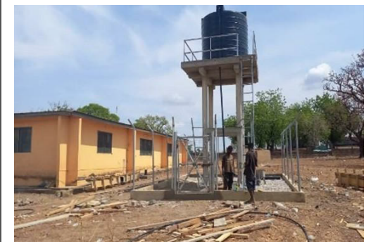
Solar-powered mechanized water system for the Tilli Health Center
