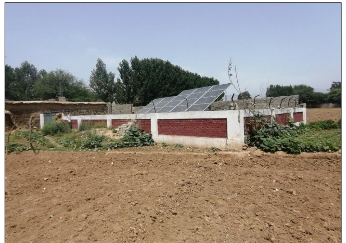
Photo 10: External view of solar panel compound – IWSS Pacha Killi, Bajaur
