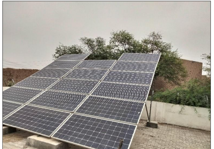
Photo 02: Solar panels installed at site – DWSS Ghundi 5 Jamrud, Khyber
