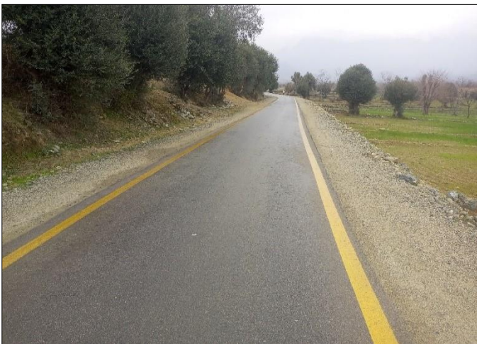
Photo 03: Asphalt wearing course completed from RD 10+000 to RD 20+000 – Loesam Nawa Pass Road, Bajaur
