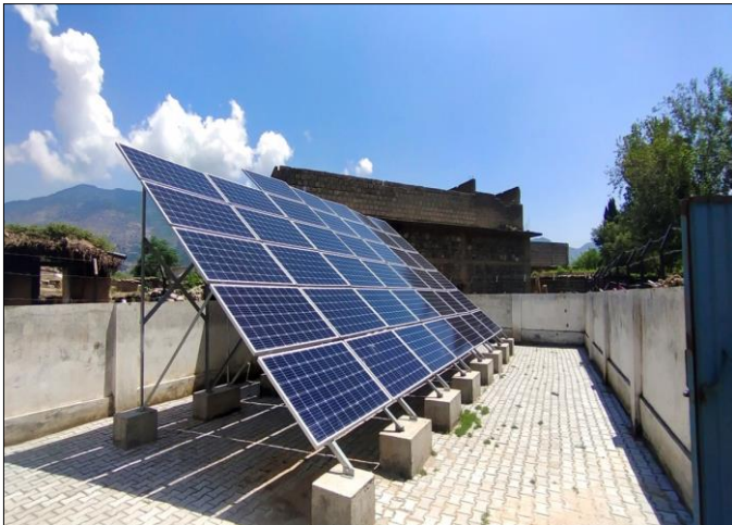
Photo 03: Solar panels installed at site – DWSS Lara Dagai Salarzai, Bajaur
