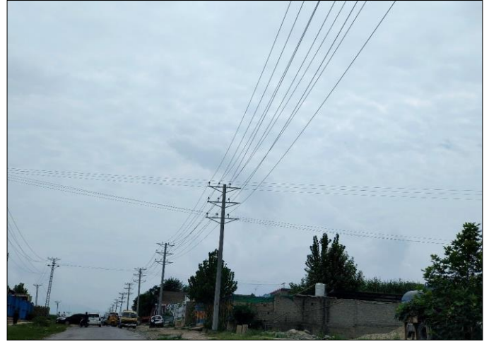
Photo 02: In progress stringing of Dog Conductor (7/0.186) at 45ft PC poles for Lagharai along with TESCO feeders – 132kV Transmission Line & 11kV Feeders Interlinking Khar, Bajaur
