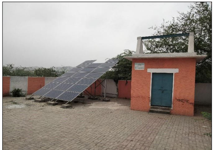
Photo 06: Internal view of solar panel compound – DWSS Godar 3 Jamrud, Khyber
