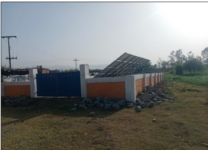
Photo 05: External view of solar panel compound – DWSS TW#07 Toheed Abad, Khyber
