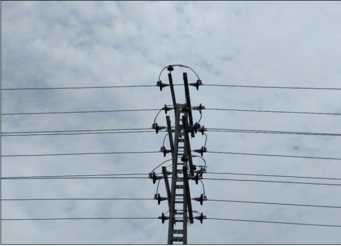
Photo 01: Newly installed disc insulators, double cross arms & Dog conductor for Lagharai along with TESCO feeders – 132kV Transmission Line & 11kV Feeders Interlinking Khar, Bajaur
