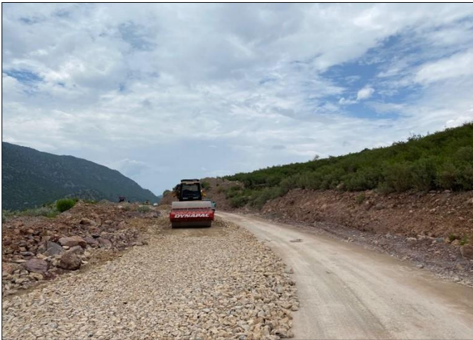
Photo 01: Compaction of water bound macadam in progress from RD 28+800 to RD 29+200 – Bara to Mastak Road, Khyber
