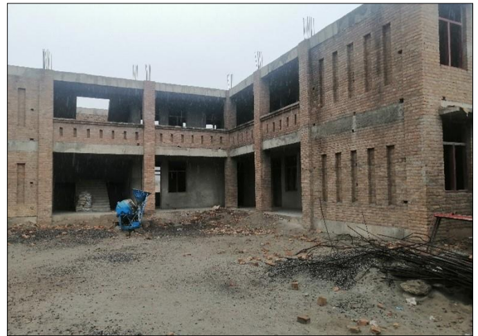
Photo 10: Construction view of main school building – GGMS Noor Ali Khel, FR Kohat
