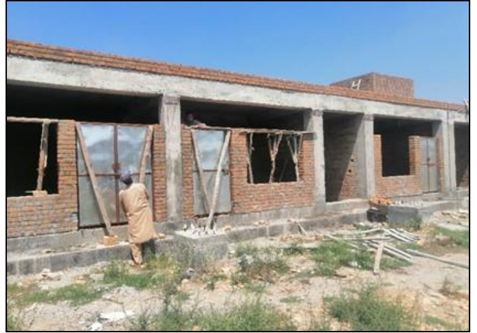
Photo 02: Steel doors fixing, and lintel beam formwork of workshop building was in progress.
