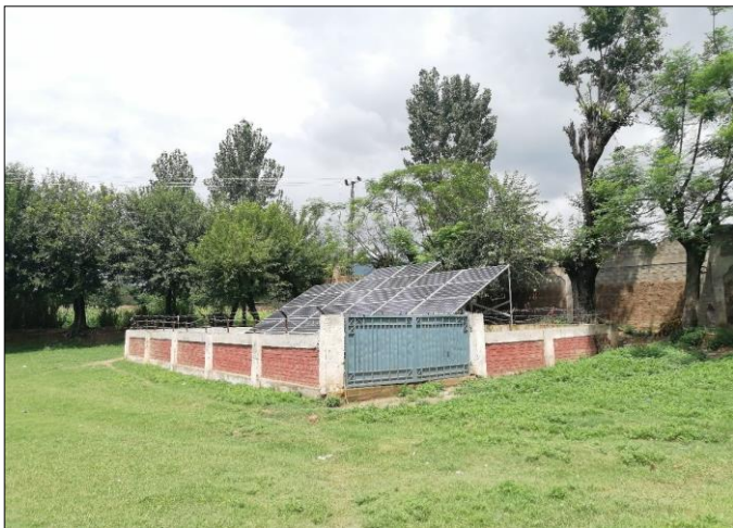
Photo 09: Solar panel compound – IWSS Zaga Dherai, Bajaur
