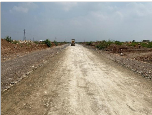
Photo 05: Water bound macadam in progress from RD 3+200 to RD 3+250 – Jamrud Bypass Road, Khyber
