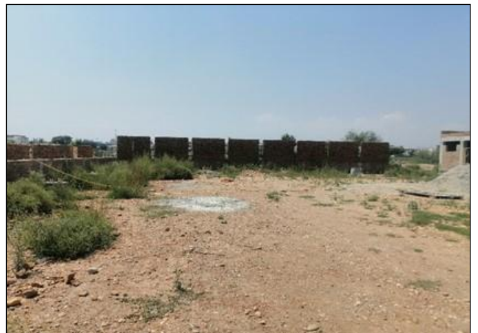
Photo 04: Brick masonry of west side outer walls of main truss workshop have been completed up to bond beam level.
