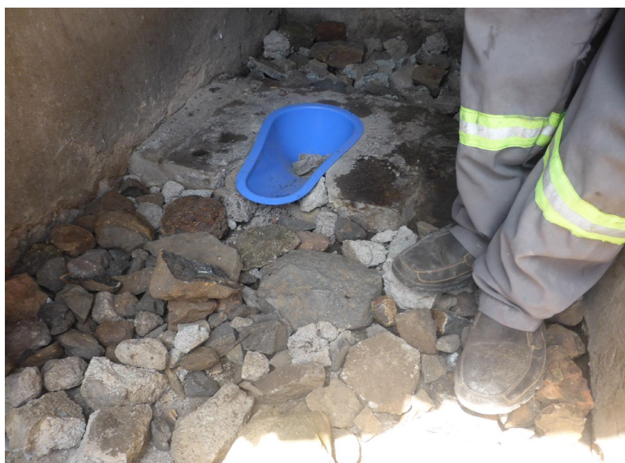
Exhibit I. The USAID WKSP-trained artisans repaired a toilet slab to fit a SATO pan. Photo: USAID WKSP
