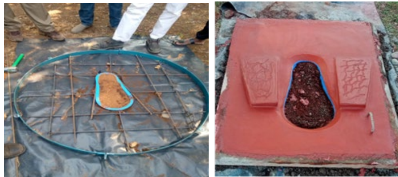
Practical session on preparation of pre-cast circular slab reinforcement and production of pre-cast circular slab with SATO
