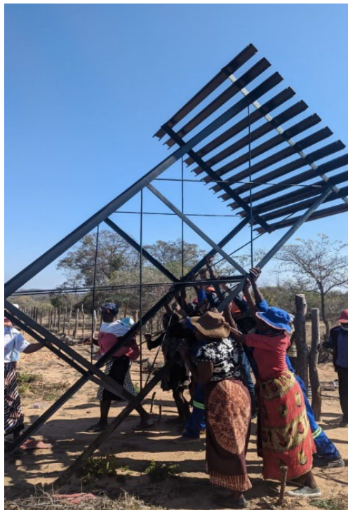
Ngwenyama farmers putting up the stand for their new water tank. Photo credit: Georgina Hove.
