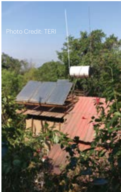
Solar water heating system
