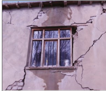
Residential Structure in Bingöl, Turkey
