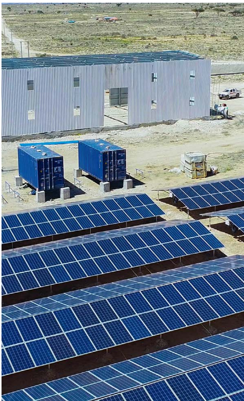
The Sanaag Electric Power Company (SEPCO) Power Station in Erigavo
