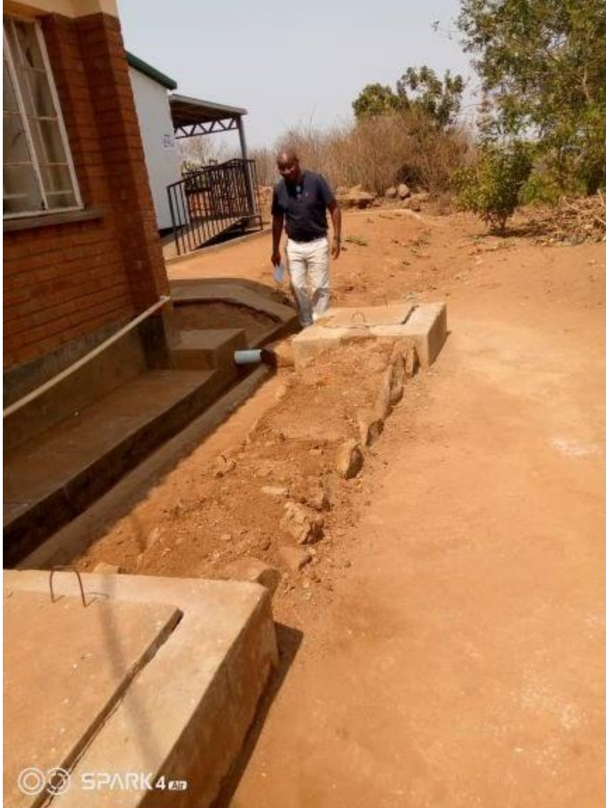
The status of the sewer pipes at Mwandama Clinic after intervention by ONSE with Sam Sande WASH Officer, inspecting the work. Photo credit Berlings Banda, Water Governance Technical Advisor
