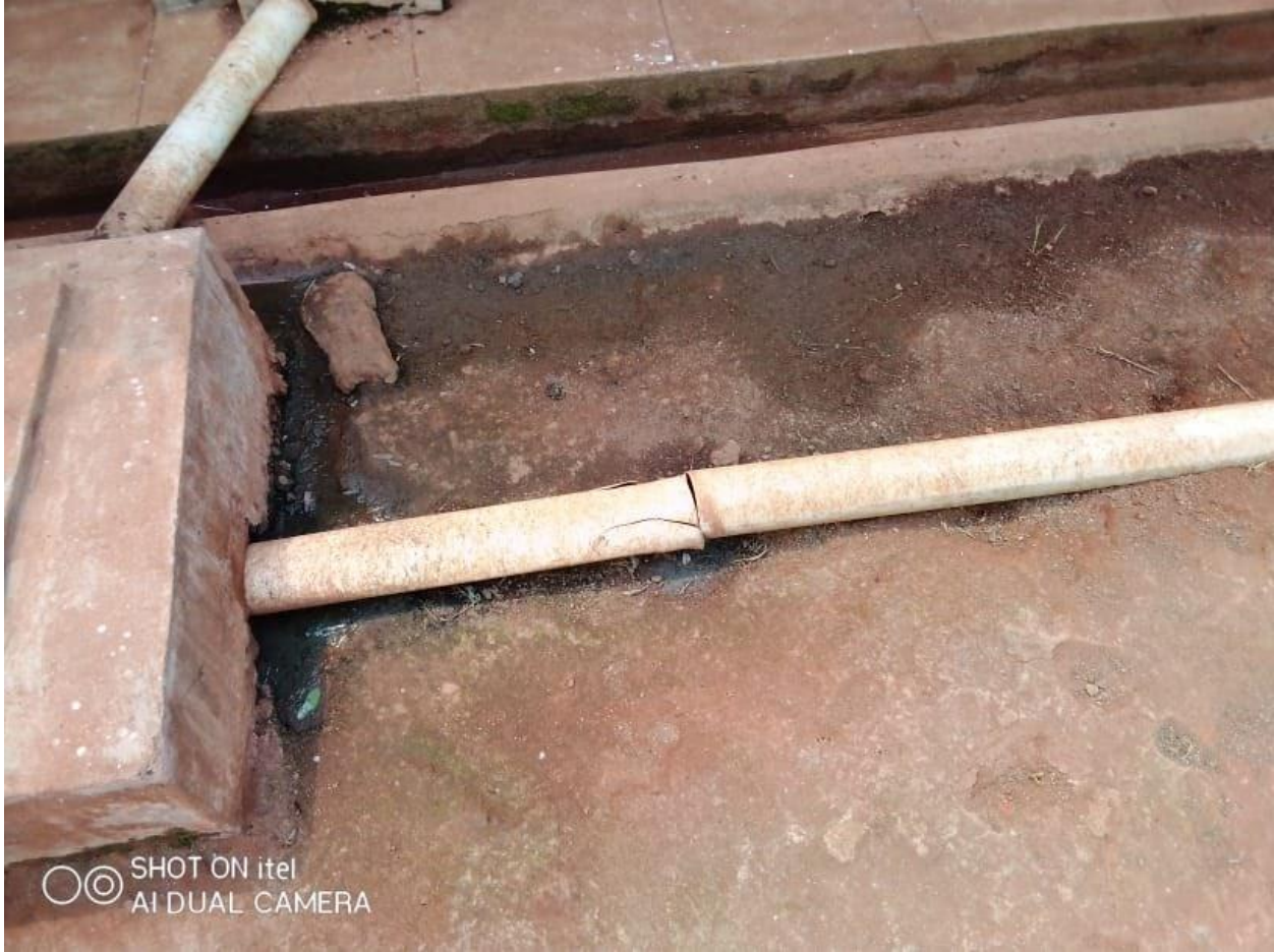
The status of the sewer pipes at Mwandama: Pic credit by Sam Sande WASH Officer - Zomba
