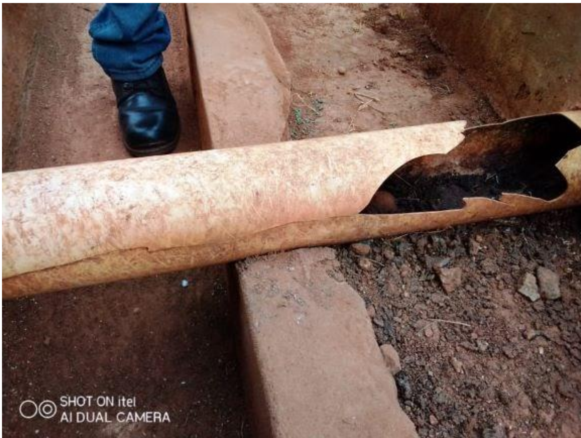
Broken sewer pipe at Mwandama; Pic credit by Sam Sande WASH Officer - Zomba
